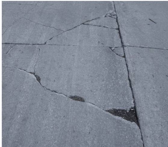
Figure 2.5: Corner cracks in concrete pavement (National Concrete Pavement Technology Center (used with permission)).
