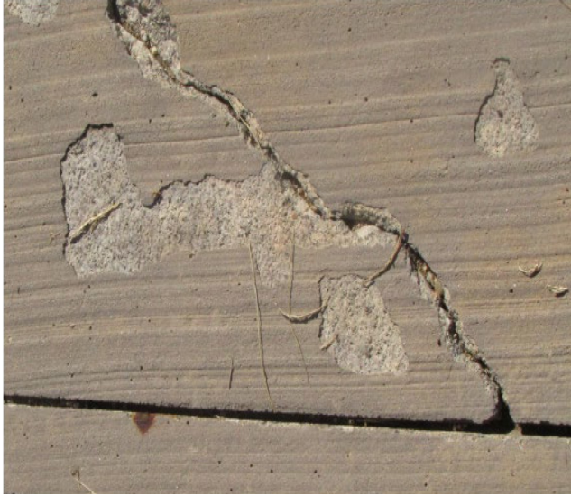
Figure 2.9: Scaling (National Concrete Pavement Technology Center (used with permission)).
