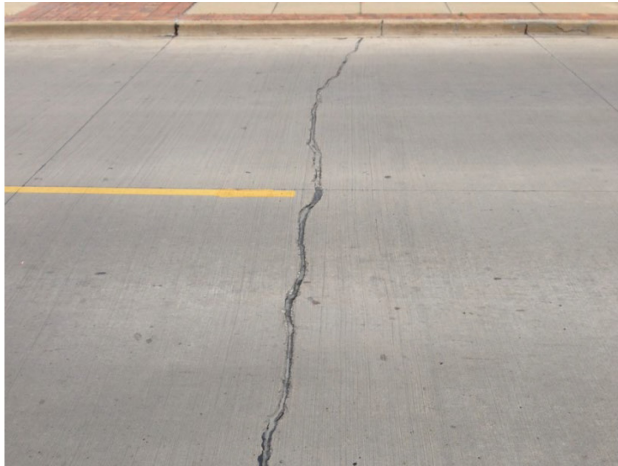
Figure 2.3: Illustration of transverse cracks on JPCP (Harrington et al., 2018).
