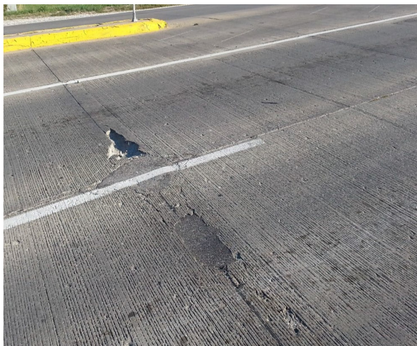
Figure 2.7: Spalling from heavy loads (Harrington et al., 2018).
