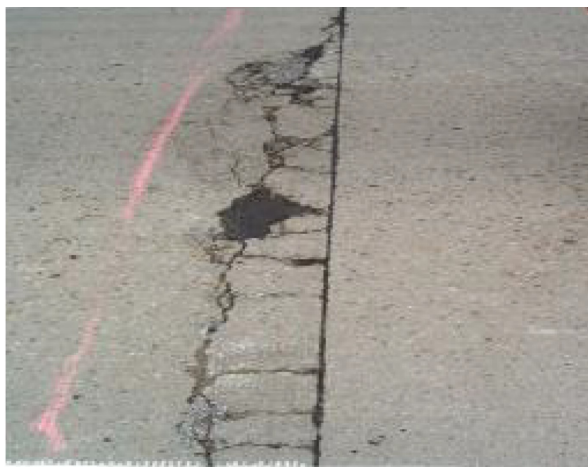
Figure 2.8: Spalling due to misaligned dowel bar (Harrington et al., 2018).
