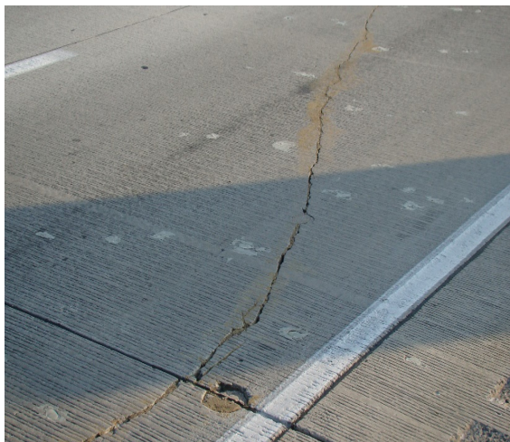
Figure 2.1: Longitudinal cracking crossing the transverse joint in JPCP (Harrington et al., 2018).
