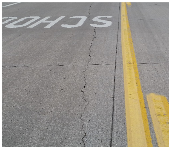
Figure 2.2: Longitudinal cracking due to delayed sawing in JPCP (Harrington et al., 2018).
